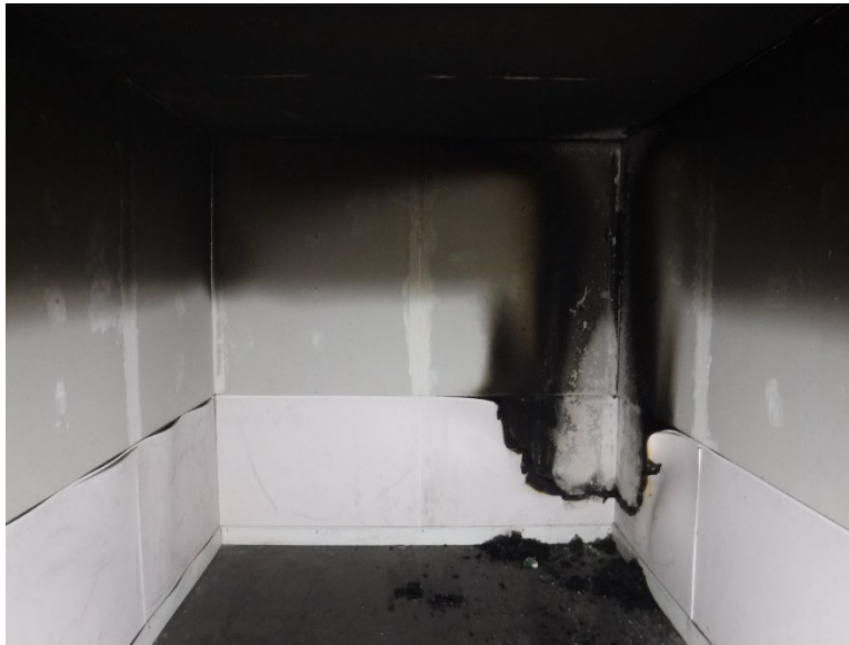
Photo No. 7 Post Test
